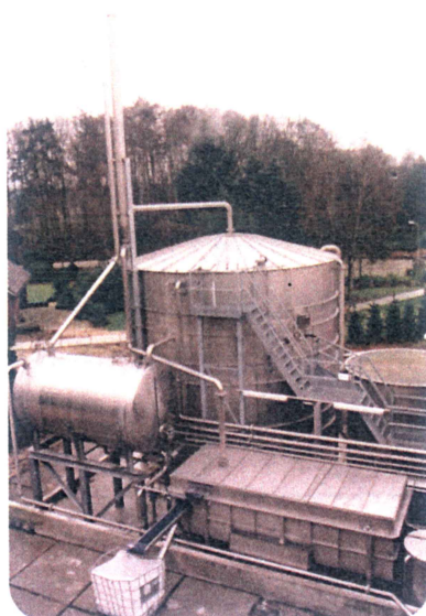
Influent tank, DAF unit and bioreactor of VHP Ugchelen.
